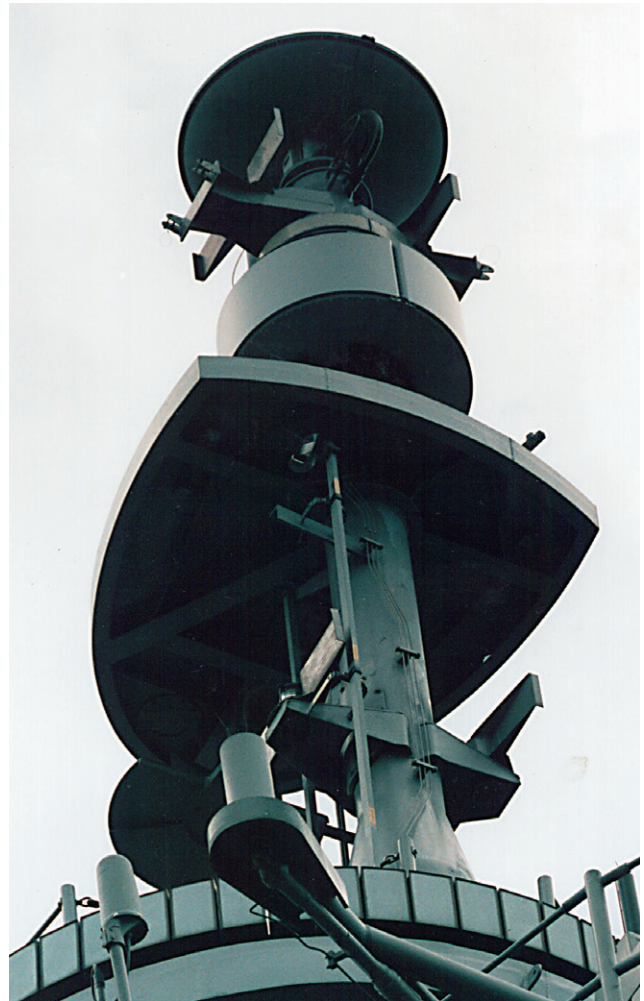
Figure 5. The DDS phased array antenna on the USS Cape St. George . The array is a 44-in.-dia. by 14-in.-high cylinder with about 1,000 array elements. It is capable of steering in both azimuth and elevation. The large structure underneath the array is an electromagnetic shield between the DDS and LAMPS antennas.
