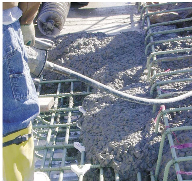
Figure 4. Deployment of WESP Smart Aggregate (WESP/SA) units in a concrete bridge deck.
