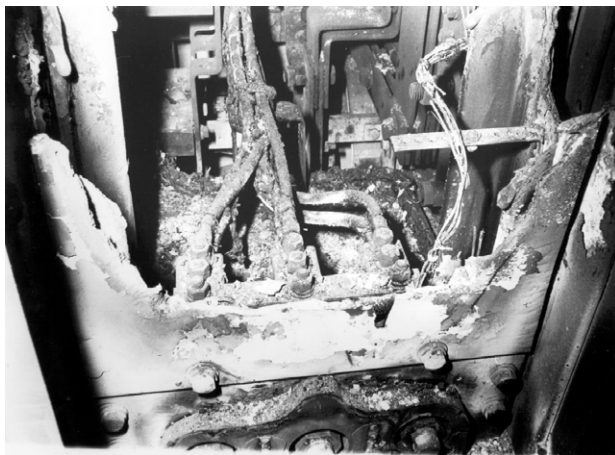
Figure 1. Arcing damage sustained on USS Parche (SSN 683). Note that some of the copper bus, cables, insulators, and switchboard structure are missing.
