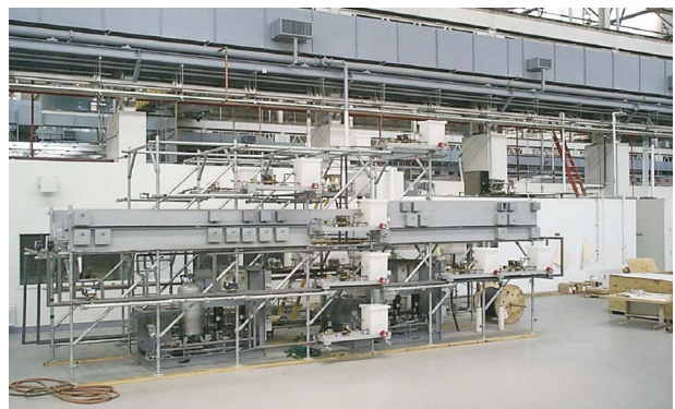
Figure 6. The chilled water testbed.
