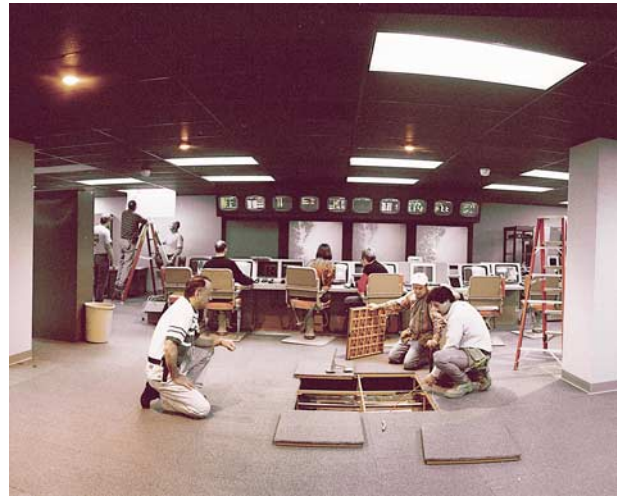
Figure 7. CSEL in Building 6 was constructed by in-house staff.
