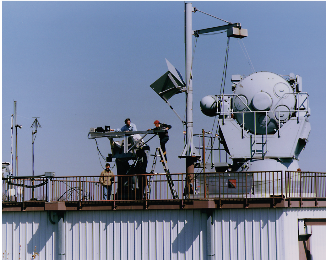
Figure 6. IR passive ranger test unit under installation in a horizontal configuration adjacent to the AN/SPG-55B radar.
