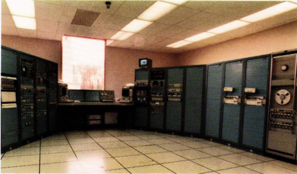
Figure 6—Operations room of the Satellite Tracking Facility.
